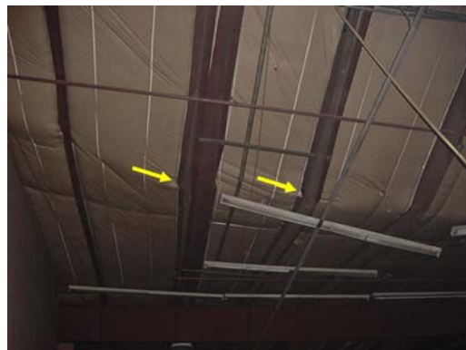
Photo 18. Failed roof - metal z-purlins rotated and buckled.
