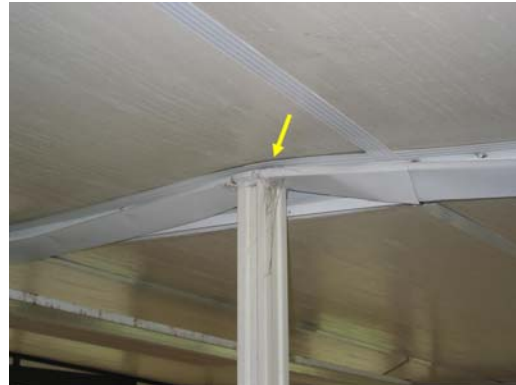
Photo 19. Crushed roof beam on prefabricated metal building.
