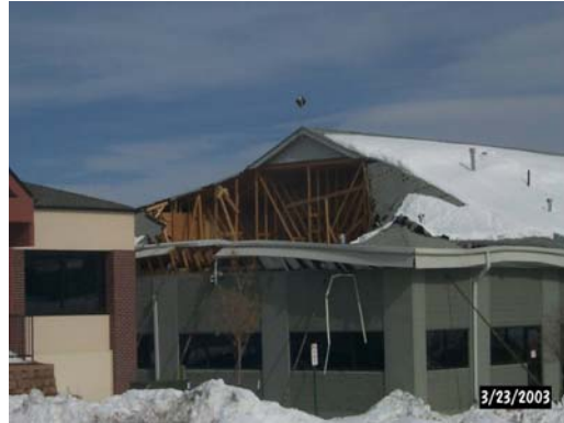
Photo 15. Collapsed roof due to snow load.
