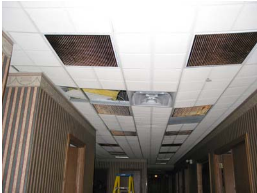
Photo 2. Deflection of suspended ceiling system.
