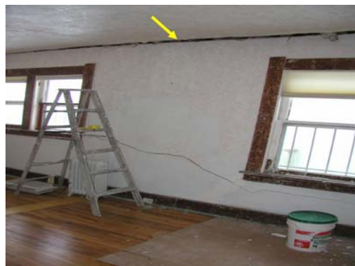
Photo 10. Gap between exterior wall and ceiling framing due to outward roof thrust.
