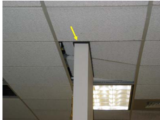
Photo 3. Incompatible deflection of ceiling system at partition wall.
