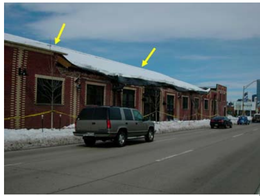
Photo 24. Photograph showing extent of damaged parapet and break line of snow slide.
