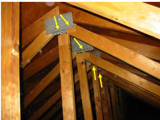
Photo 13. Truss web pull-out from press plate at panel point connection.
