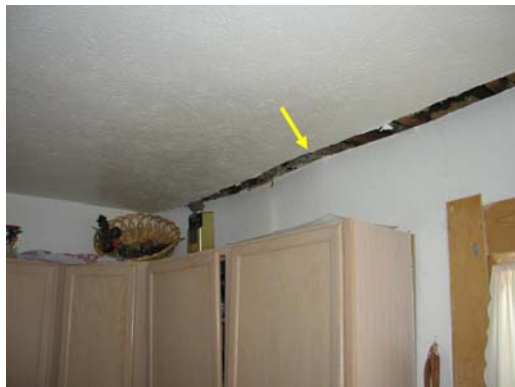
Photo 9. Gap between exterior wall and ceiling framing due to outward roof thrust.
