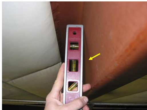
Photo 16. Deflected/rotated metal z-purlin.
