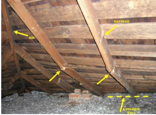
Photo 6. Cracked roof rafters in a Denver Bungalow.
