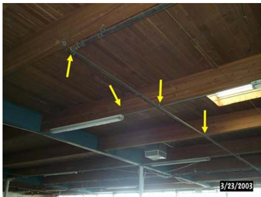
Photo 4. Utility line endangered by damaged roof beam.
