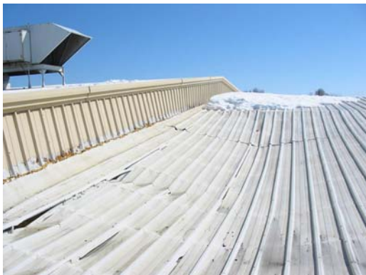
Photo 17. Failed roof over metal z-purlin supports.
