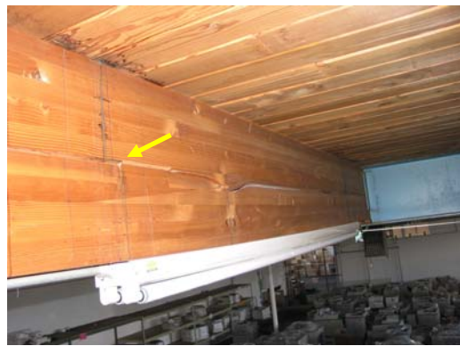
Photo 20. Shear crack parallel to grain in glued laminated timber beam.
