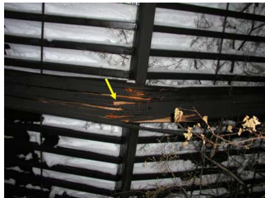
Photo 21. Failed trellis roof structure due to snow "bridging" the gaps between roof members.
