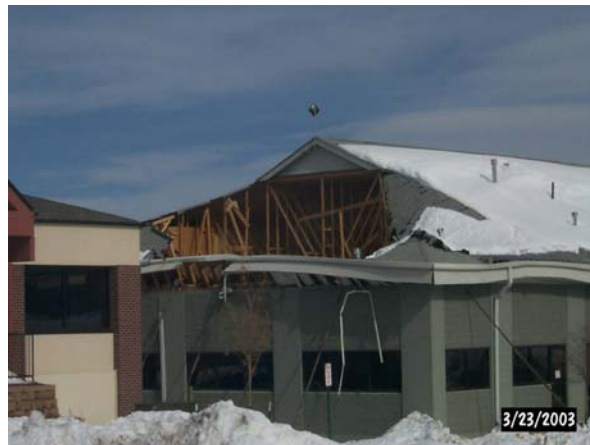
Photo 1. Collapsed roof due to snow load.
