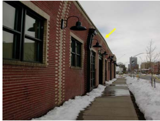
Photo 22. Parapet wall bowing outward under lateral forces from snow build-up behind the wall.
