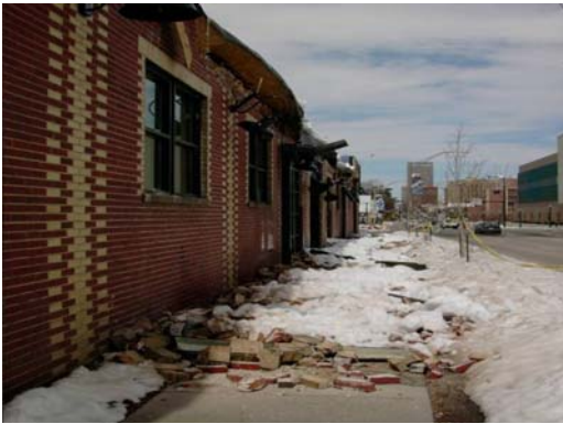
Photo 23. Failure of a section of parapet wall.
