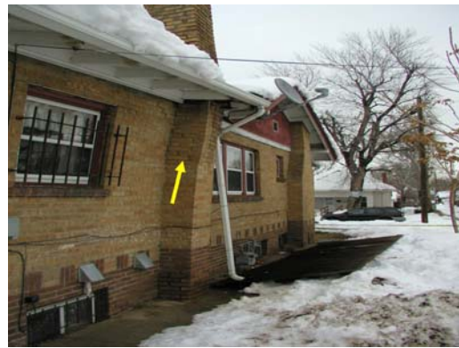
Photo 8. Leaning brick on exterior wall of a house due to outward roof thrust.
