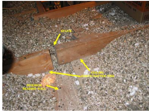
Photo 12. Splice of ceiling joists being pulled apart by outward roof thrust.
