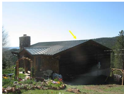
Photo 25. House with standing seam metal roof and no snow guards.
