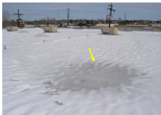
Photo 5. Ponded water on warehouse roof.
