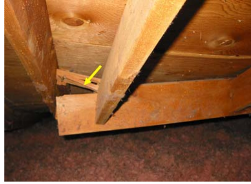
Photo 7. Damaged roof connection of a Denver Bungalow.
