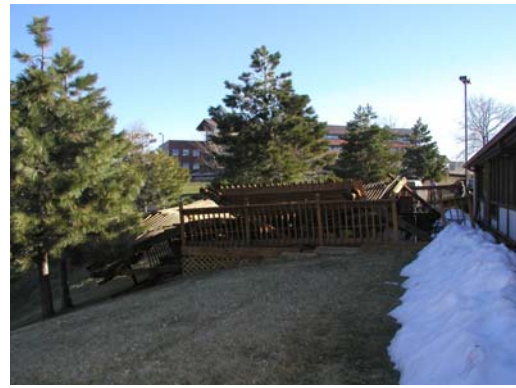
Photo 27. Lateral collapse of trellis structure due to sliding snow.
